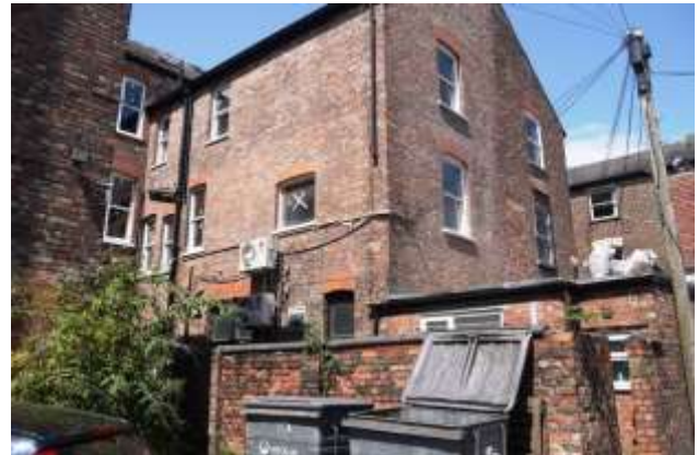
Typical issues to the rear of properties including vegetation growth, air-conditioning units, bins and brickwork in poor condition.
