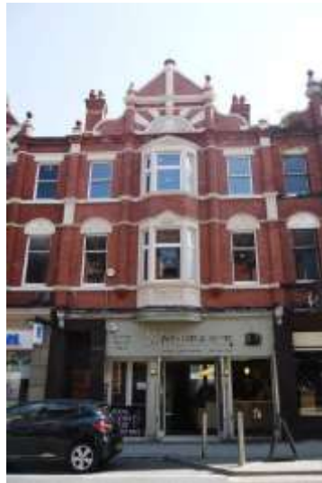
Good example of a well-maintained property (31 Stamford New Road). However the stone work has been inappropriately painted
