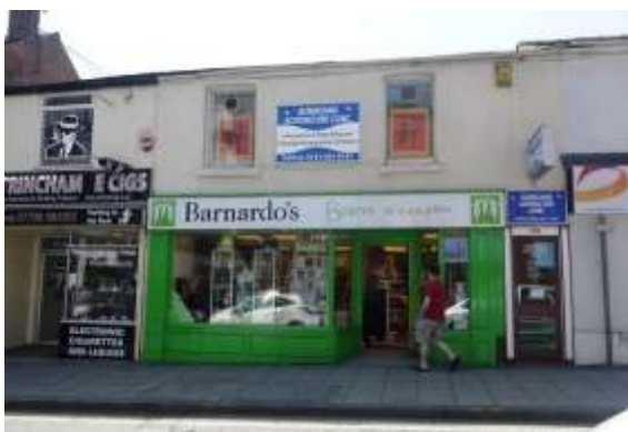
Traditional shop front, harmed by surrounding inappropriate advertising and modern signage, particularly on the upper floors.
