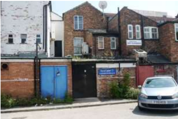
Rear of Stamford New Road, within Lloyds Square, showing intrusive air conditioning units and some painted rear elevations.
